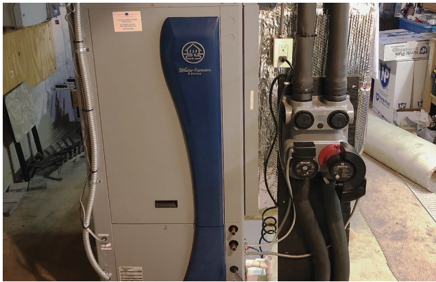
Ground-source heat pump indoor unit
