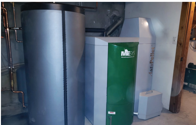
Biomass heating indoor unit
