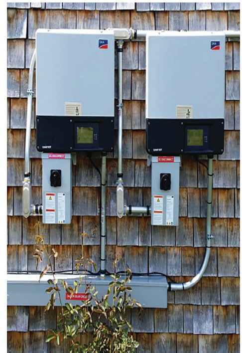
Inverters installed outside of residence
