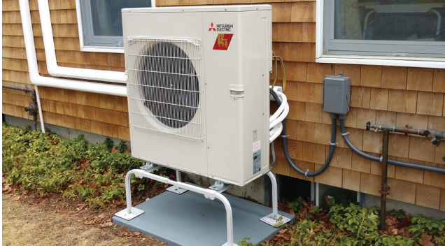
Air source heat pump external unit
