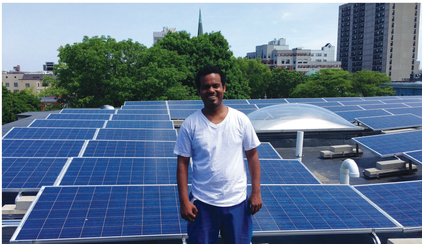
Solar electric system on multi-family flat roof building
