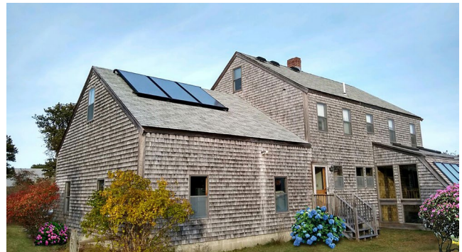
Solar hot water system
